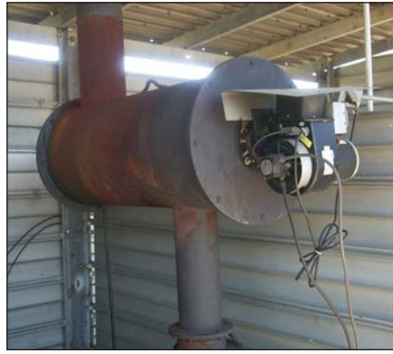
Figure 2. An afterburner used for a more efficient burn of exhaust gases.
