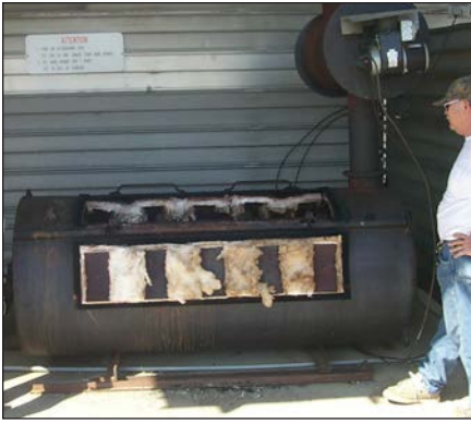
Figure 1. An example of an incinerator with an afterburner.
